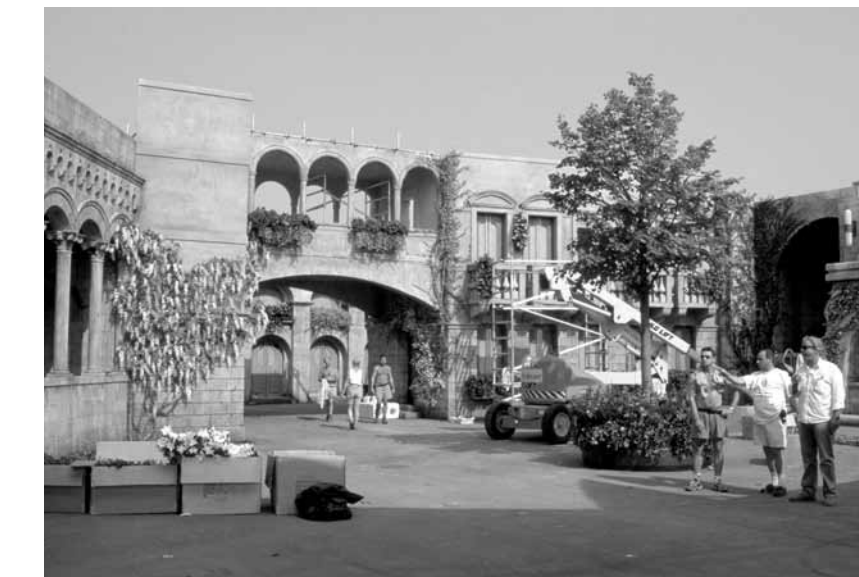
ABOVE Creating the set dressing of the Theed Plaza on the backlot at Leavesden, early summer 1997 (the upper portions of the buildings would be added digitally by ILM in post); dressing/props charge hand Peter Watson, dressing props supervisor Martin Kingsley, and set decorator Walpole.
